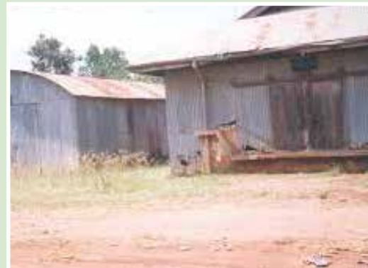
Dilapidated Facilities that was used for storing obsolete chemicals in Kawanda, 2005
